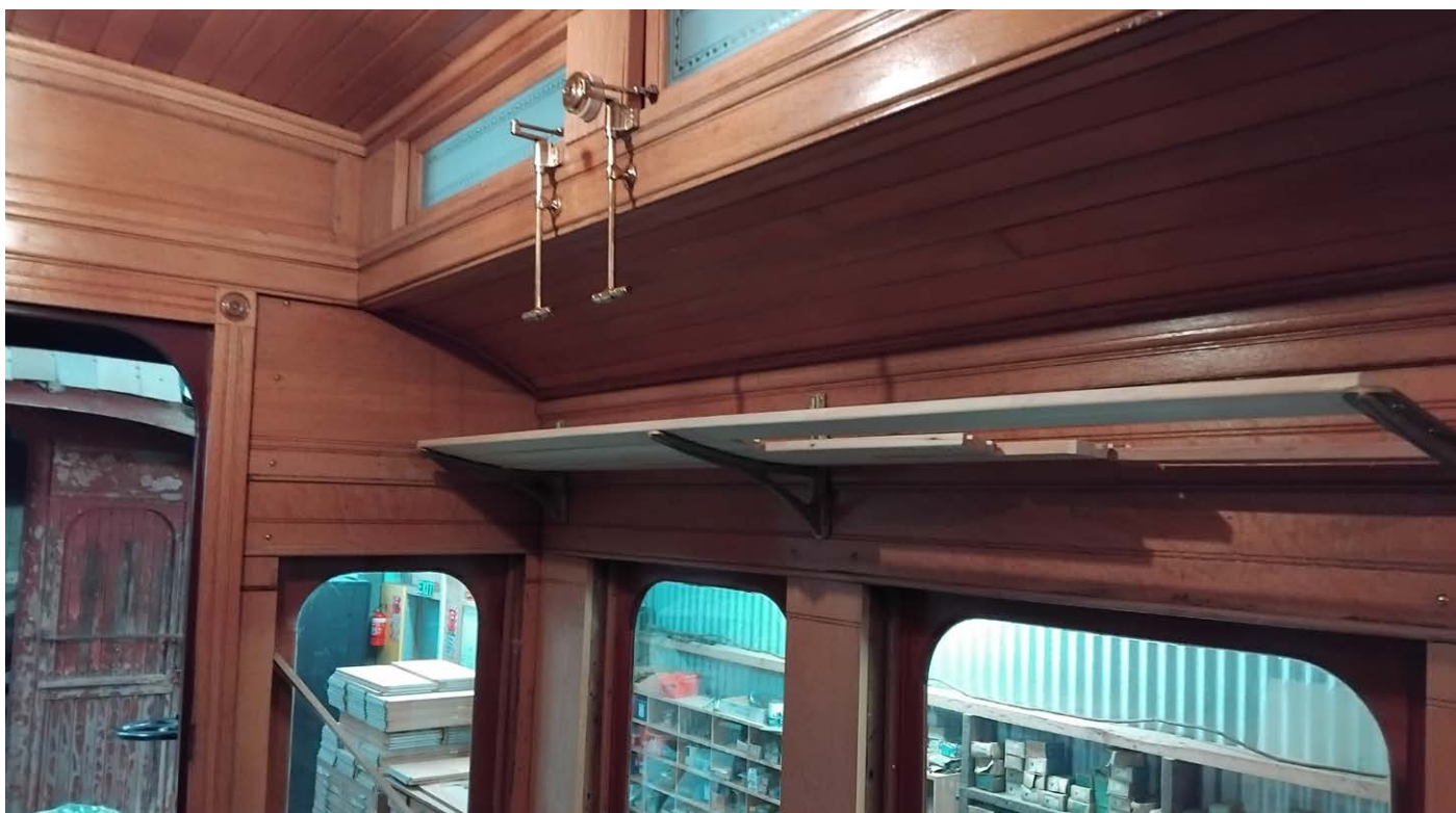
Finishing work is well in hand inside the saloons of WMR car 48. The electric lights work and the oil lamps are ready for installation after other interior work is completed. Shown here is the fitting of brackets for the luggage racks and the beginnings of woodwork for the racks. WMR carriages had wooden slatted racks, different from NZR's pipe and netting racks. Photo: Rob Merrifield
